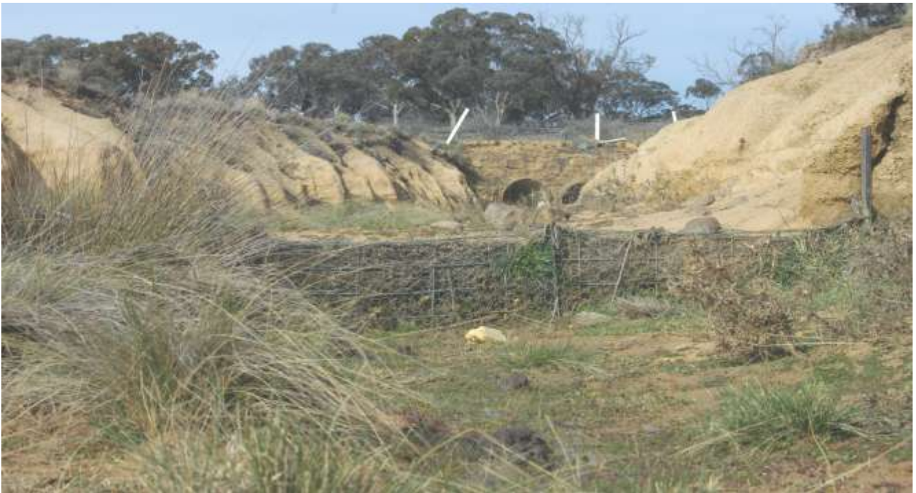
Figure 15: This sediment trap at Kangaroo Ground has reached capacity and is in need of replacement. Again note the effectiveness of the trap in mitigating sediment and elevating the level of the gully floor. Revegetation is better able to establish on the trapped sediment, especially where stock access is managed.
