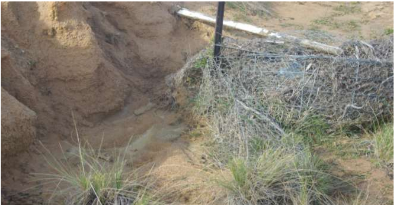
Figure 16: As well as reaching capacity, many sediment traps have minor repair issues. Most have occurred where built up sediment and debris obstructs the flow of water after a rainfall event; an alternative pathway then erodes the weakest point of the structure, usually at the side (as is the case above). Although reducing the overall effectiveness of the structure, it is not of significant concern, (especially given the large number of structures) except where concentrated flow causes bank scouring.
