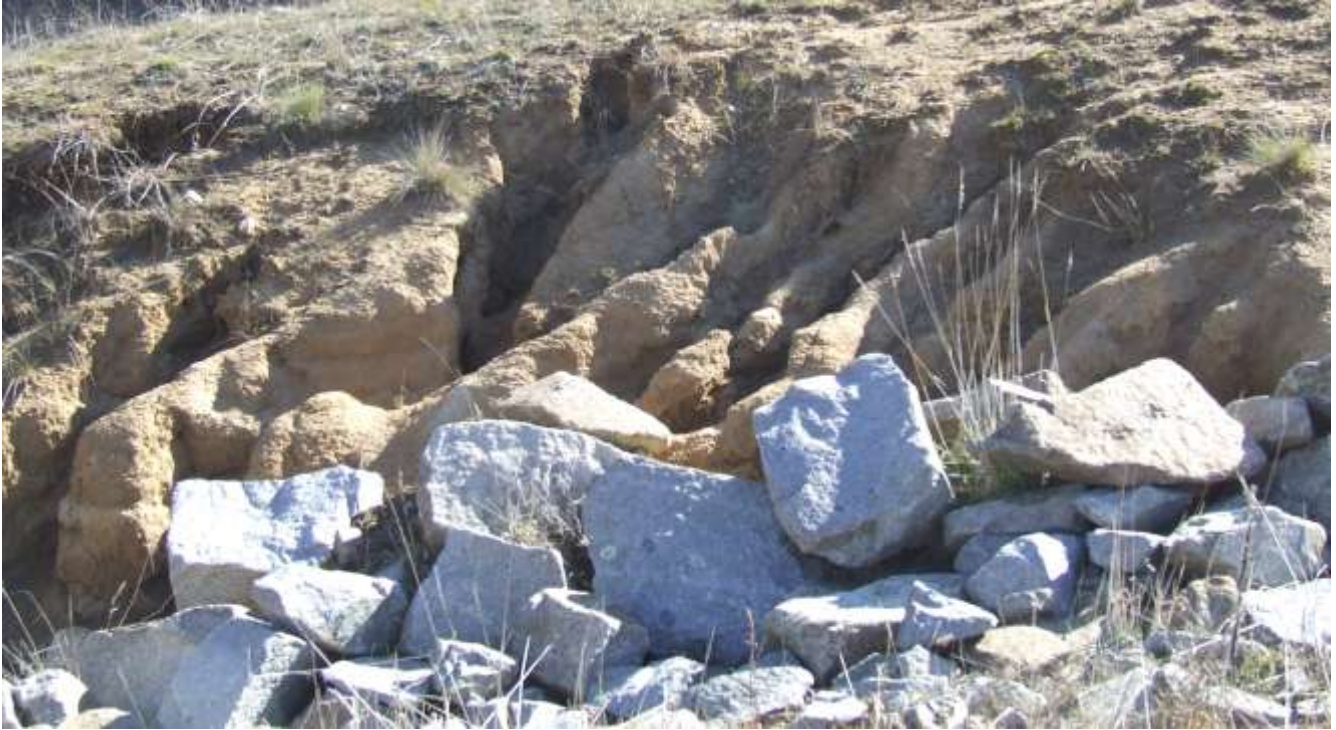
Figure 34: The outer edge of a rock flume at Ron Reed's property Woodborough. Overland flow has eroded along the edge of the rock armour causing further erosion.
