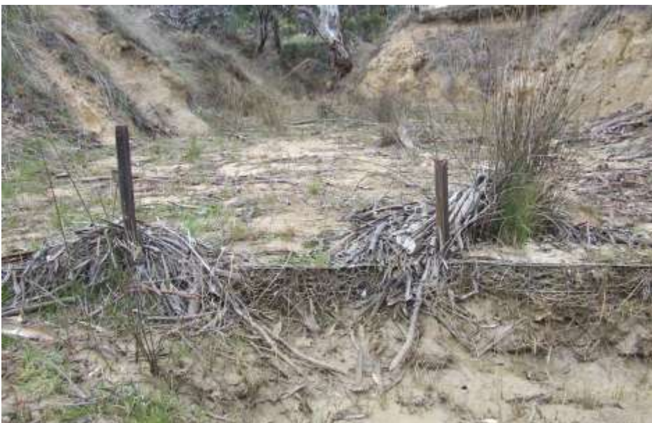
Figure 14: Wire mesh weir at capacity at Hollyridge. Again note the elevation of the gully floor with retained sediment (figure Emma Platts 2007).
