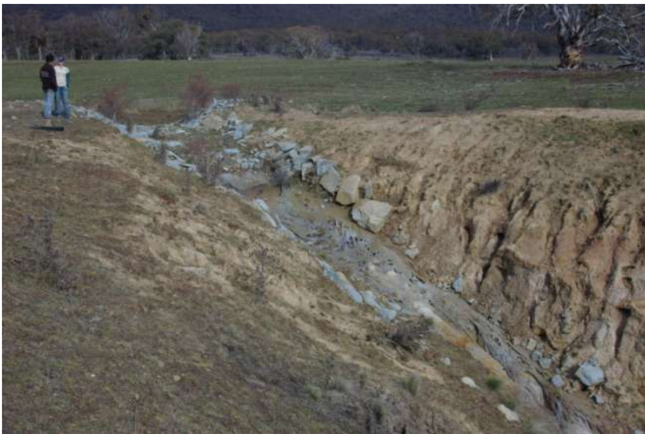
Figure 26 (below): Greg Walker (landowner) and Emma Platts, discuss a failed flume at Avondale. This failure was due to inadequate rock size combined with too steep batter grades. Note the movement of rock and the exposure of geotextile. The batter banks are actively eroding as a result (figure courtesy Emma Platts 2007).
